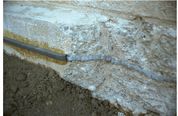
Rough Concrete Cold Joint
