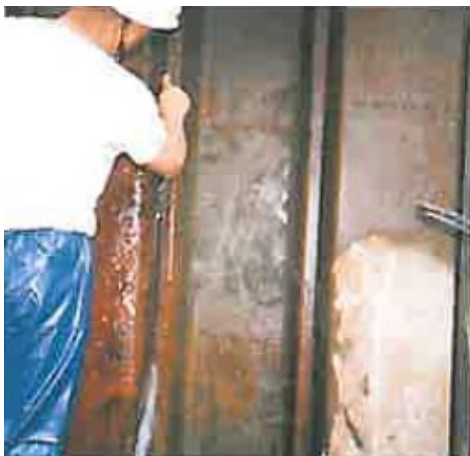
State of water leakage
